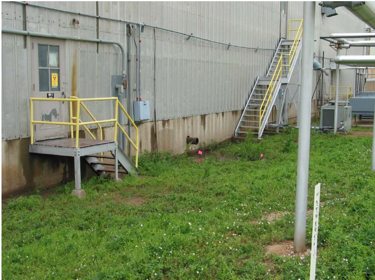
Figure 3– Side View of Building Showing Drainpipe and Flagged Sample Locations
